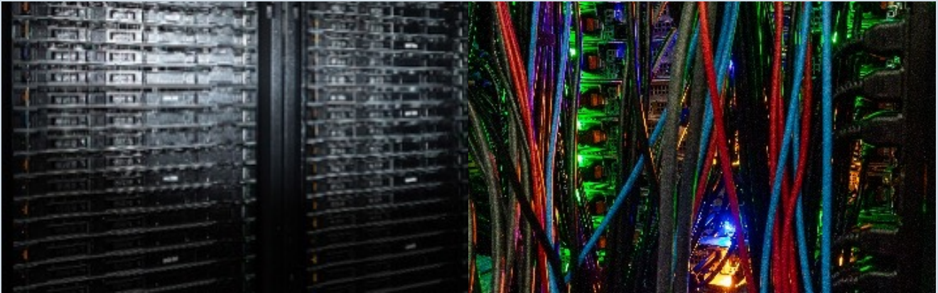
Figure 39: FLF HPC “Deep Thought”. Front of HPC racks (left) and rear of the racks (right).
